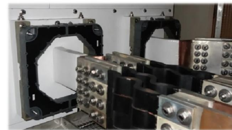
Current sensors on terminals
